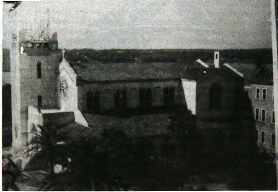
Saint Leo Abbey Church under construction in 1943. The bell tower had yet to be completed. Photo courtesy of Abbey Archives.
